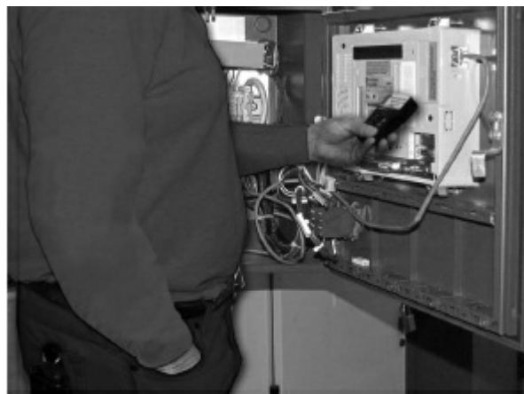
Figure 3.2 — Keep one hand in a pocket or behind your back when testing energized equipment to avoid creating a path for shock current.
