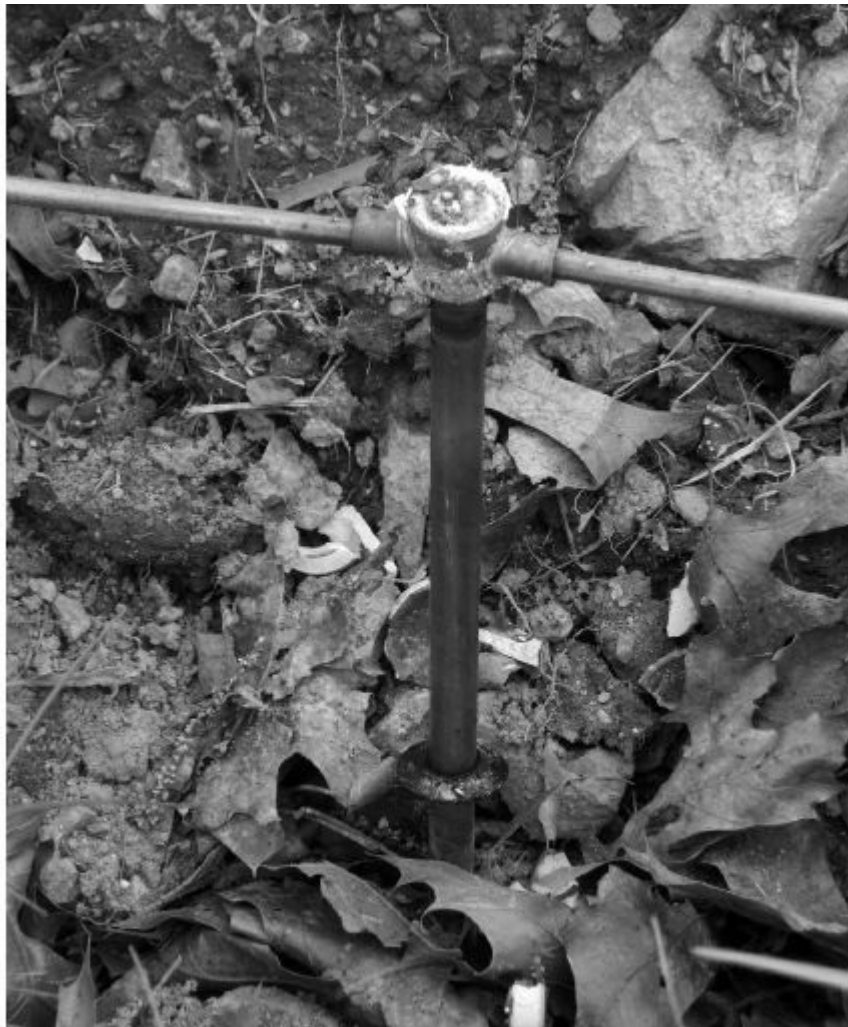
Figure 6.3 — A welded ground rod connection between #2 AWG copper wire and a ½-inch ground rod. This connection was then buried as part of a tower grounding system.
