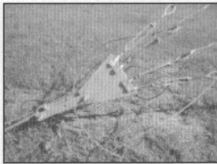
Guy wires terminate at their lower end at equalizer plates that are attached to their respective guy anchors.
