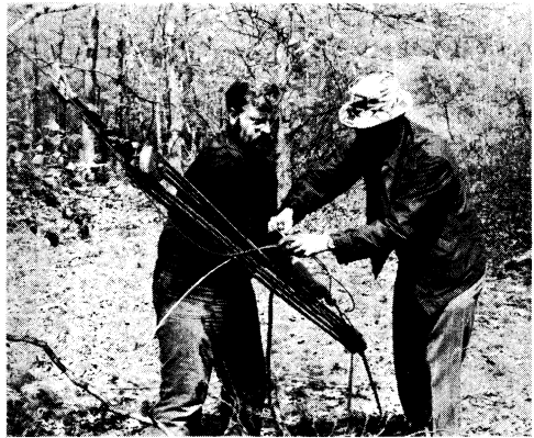
Fig. 14-11 – Proper tension can be placed on the guy wires with the aid of a block-and-tackle system. (Photo by K1THQ)
